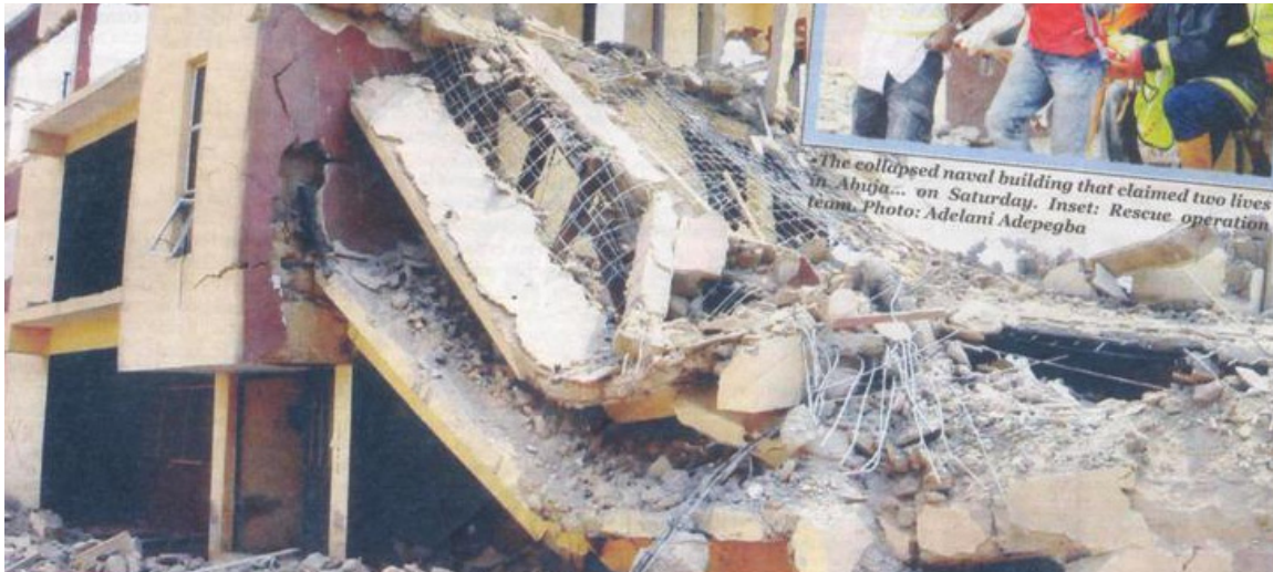
Figure 3: Building collapse as result of engagement of quacks/non-professionals (Source: Sunday Sun Newspaper' of January 29, 2012)
